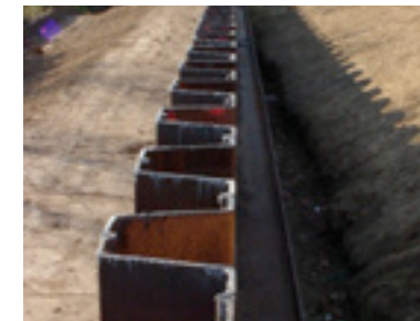
Used metal sheet piling from other Alberici job sites was used to reshape the landscape for stormwater mitigation.
